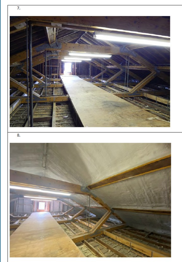
Town House 2023 Attic Insulation
